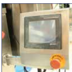
HMI control screen
