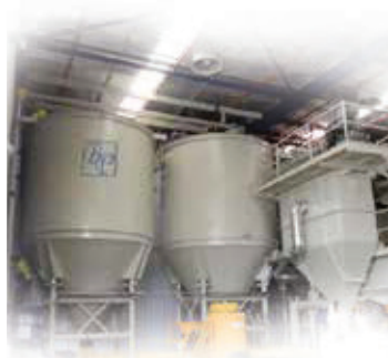
Silo / Hopper Plant Receiving System
