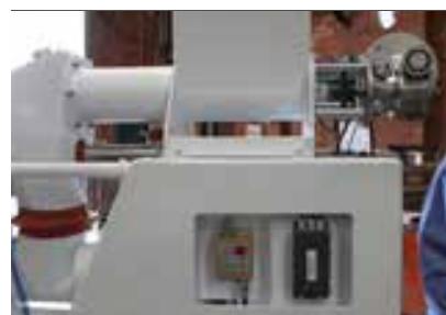
Vibratory Controls & Summation Box
